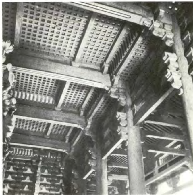
9. Ceiling of the Golden hall (Kondō) of the Shingon temple Tôji (= Kyōgokokuji), Kyoto.
