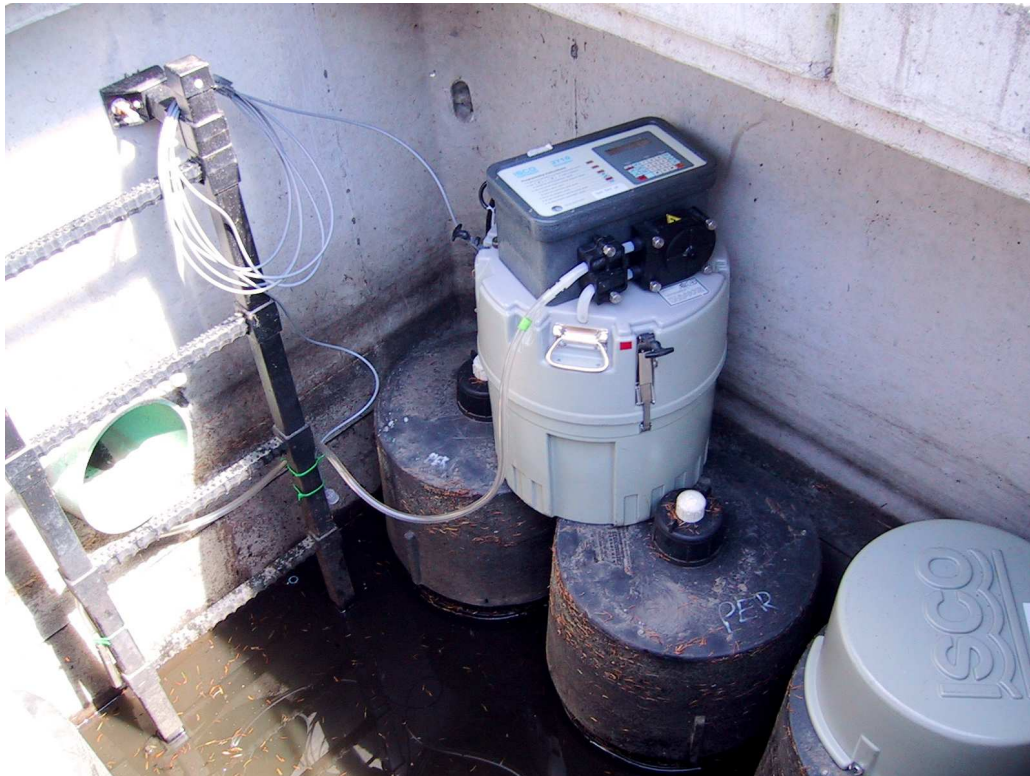
Figure A10: Photograph of the Silvern storm water treatment vault, May 2004. This site was not sampled in 2005.
