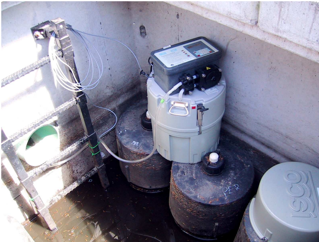
Figure 38: Silvern storm water treatment vault, May 10, 2004.
