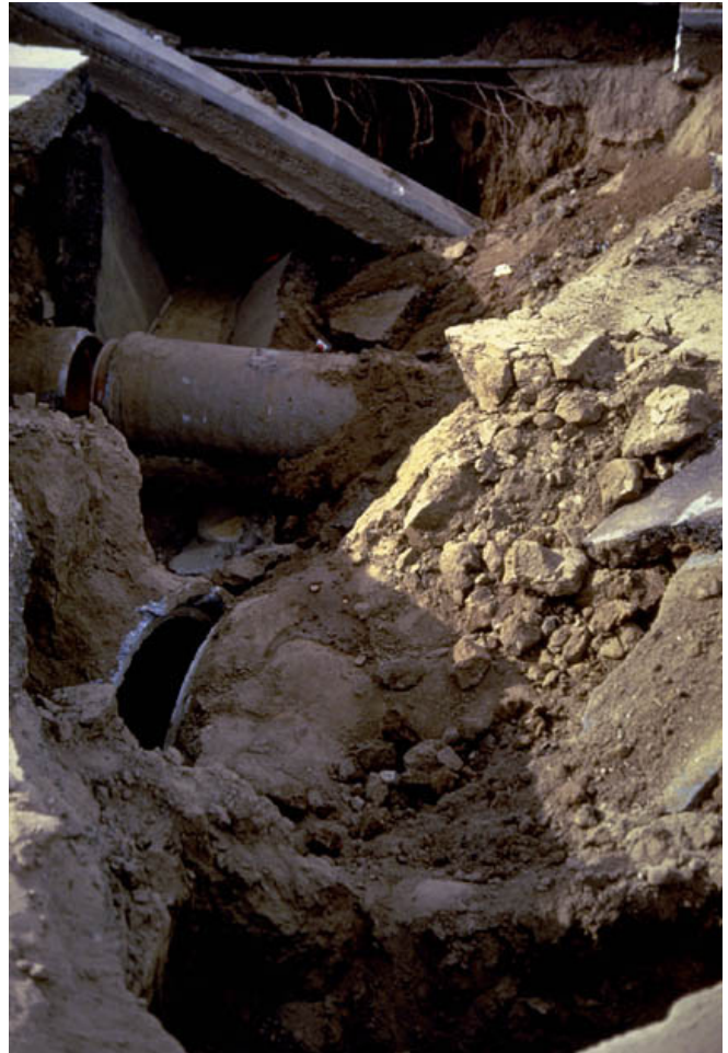
Figure 95. Pipes carrying potable water may be damaged or contaminated, leaving many survivors without a critical resource. Breaks in wastewater pipes can confound this issue, causing sewage backup into streets, plumbing, and other damaged pipe infrastructure. Photo: Vitelmo V. Bertero.
