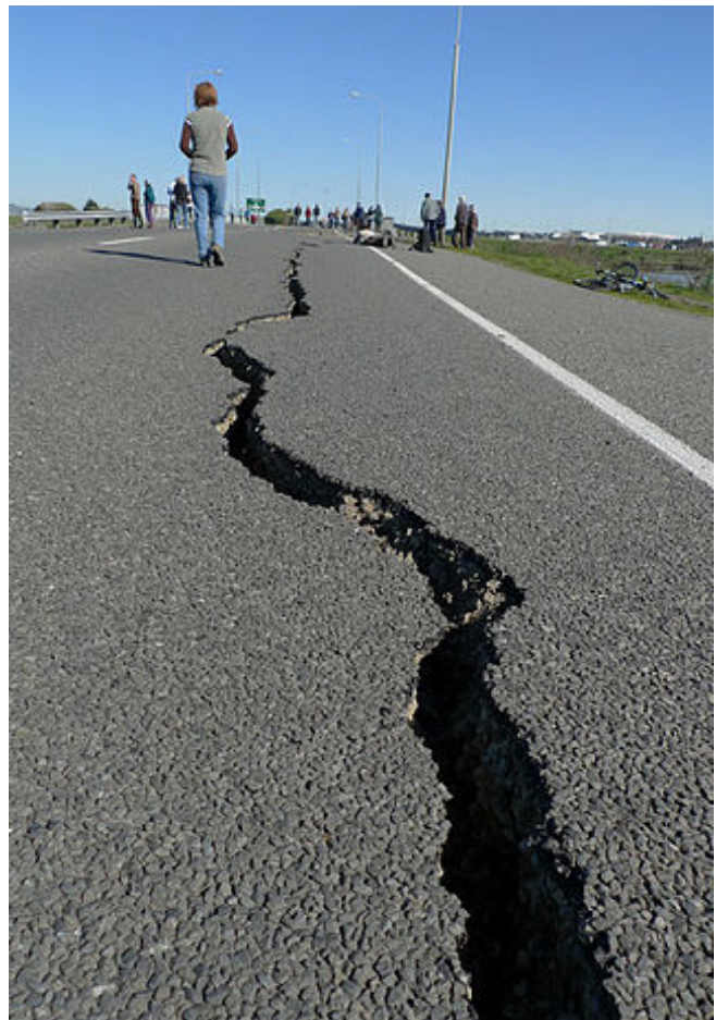
Figure 18. The 2010 M7.1 Canterbury, New Zealand earthquake caused low to medium damage to roadways, with two to five inches of permanent ground displacement. Photo: Martin Luff.
