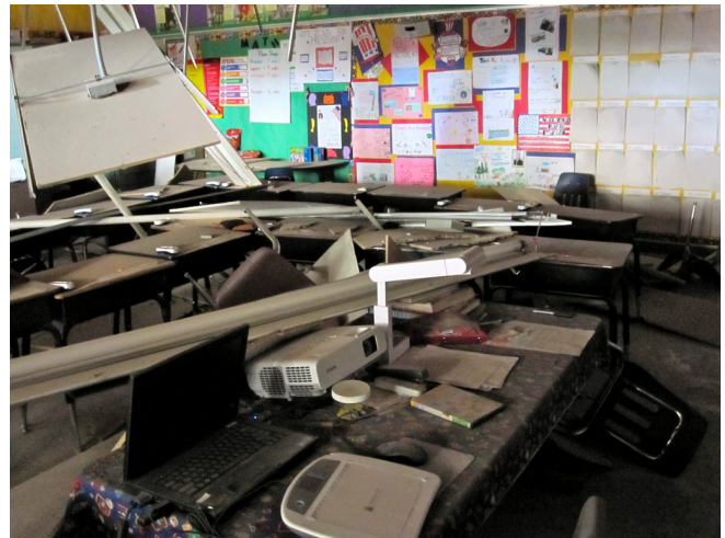
Figure 88. The 2010 Baja California M7.2 earthquake caused extensive damage to Jefferson Elementary School in Calexico, California, such that the school was closed for the remainder of the semester. Interior damage and fallen items could injure or kill students and faculty. Photo: Kelly B. Hutson.
