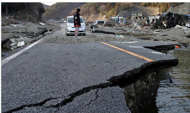
Figure 17. The 2011 Tohoku tsunami caused high damage to roadways, shifting parts of the road up or down by more than a foot. Photo: Japan Red Cross Society, published in the New York Times March 24, 2011.
