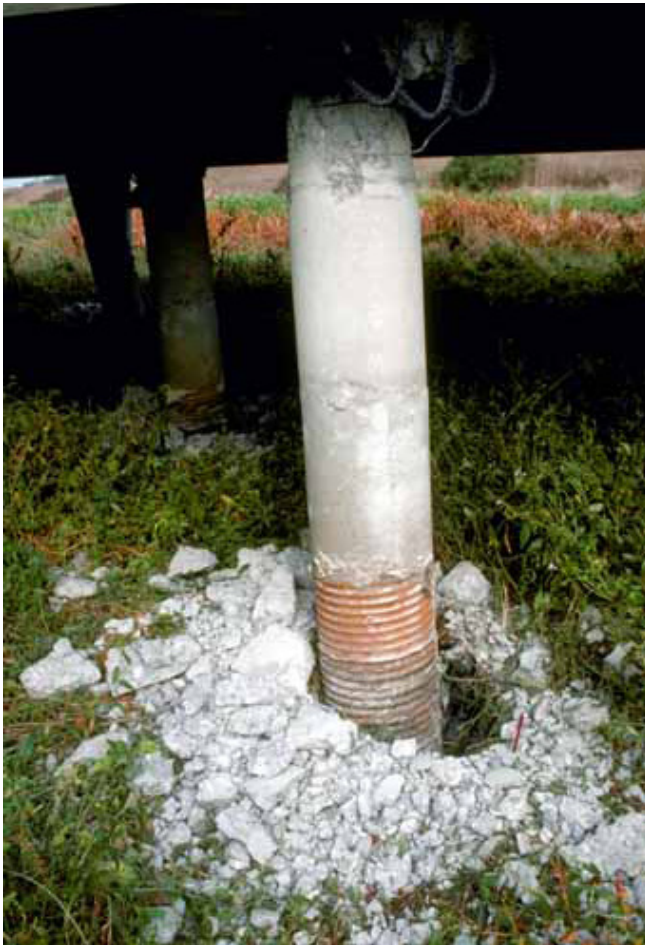
Figure 24. The 1989 M6.9 Loma Prieta earthquake in California caused medium damage to the support column of a bridge. The shaking caused the concrete to break up and shift the bridge column alignment. Photo: H.G. Wilshire, USGS.
