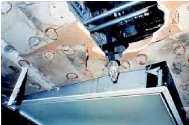
Figure 79. A hospital in Sylmar, California only suffered minor structural damage from the 1994 Northridge earthquake. However, a broken sprinkler pipe caused water damage to the hospital. This type of damage can force hospitals to temporarily shut down. At another facility, a damaged water tank on the roof leaked up to two feet of water at some locations. Photo: FEMA.
