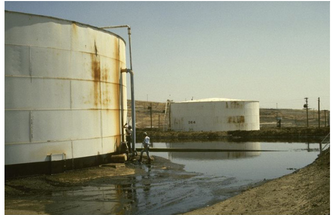
Figure 100. Shaking from the 1983 M6.5 Coalinga earthquake caused the pipe connections to break at a Chevron facility. Oil spilled out of the damaged connection, but was retained by dikes. Photo: Karl V. Steinbrugge.
