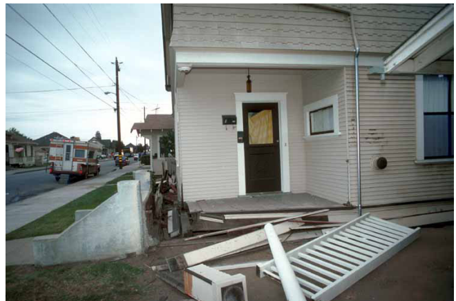
Figure 114. The 1989 Loma Prieta earthquake shifted this house over two feet off its foundation causing the structure to detach from the concrete stairway and collapsing all four shear walls. Photo: J.K Nakata, USGS.
