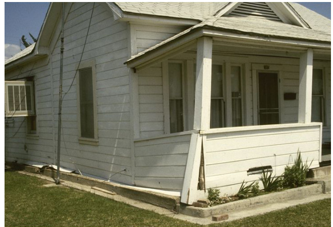
Figure 113. The 1983 M 6.2 Coalinga earthquake caused the cripple walls of wood-frame houses to fail, resulting in the house sliding off its foundation. Wood frame houses are flexible enough that collapse is unlikely for most of them, but many built prior to 1976 are at risk of shifting off of their foundations. Photo: Karl V. Steinbrugge.
