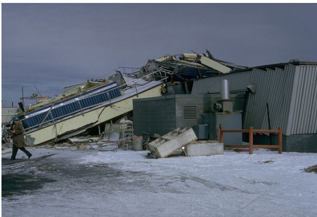
Figure 36. The Great Alaskan Earthquake in 1964 caused this reinforced concrete-framed control tower to collapse at the Anchorage International Airport. Photo: Karl V. Steinbrugge.
