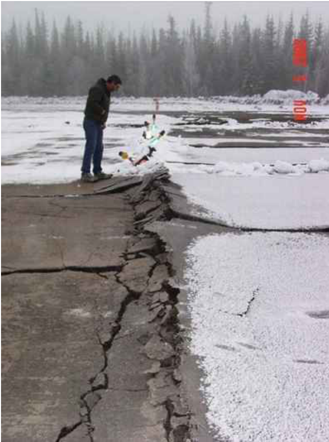
Figure 38. The M7.9 Denali earthquake in 2002 caused significant damage to the only runway at the Northway, Alaska airport. The runway was temporarily replaced with a gravel surface before permanent repairs. Photo: Unknown.
