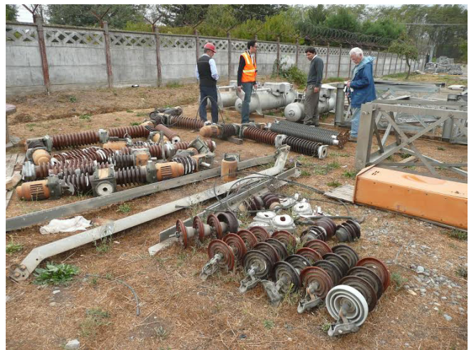
Figure 56. Earthquake damage to substation equipment. Photo: BPA Energy
