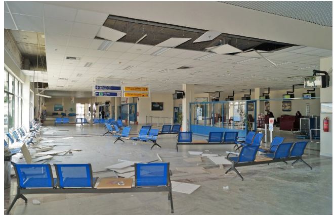
Figure 37. In 2014, a M6.9 earthquake near Greece caused nonstructural damage to airport at Lemnos International Airport in Lemnos, Greece. Photo: Ayis Theos.
