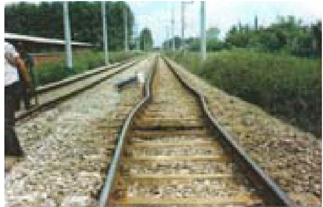
Figure 42. The M 7.4 earthquake in Turkey caused localized bending of the rail tracks. Photo: Turkish State Railways.
