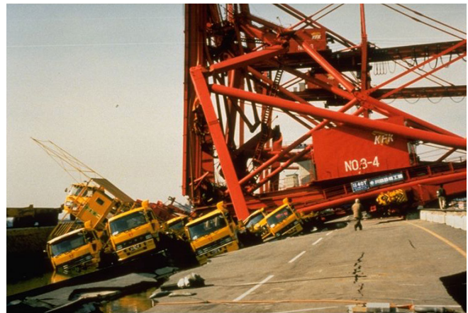
Figure 53. The 1995 M6.6 Kobe earthquake damaged a loading ramp structure at Higashi-Kobe ferry pier, along with other port infrastructure in the area. Damage to ferry facilities could isolate island populations in the San Juan Islands and slow transportation across the Puget Sound. Photo: unknown.
