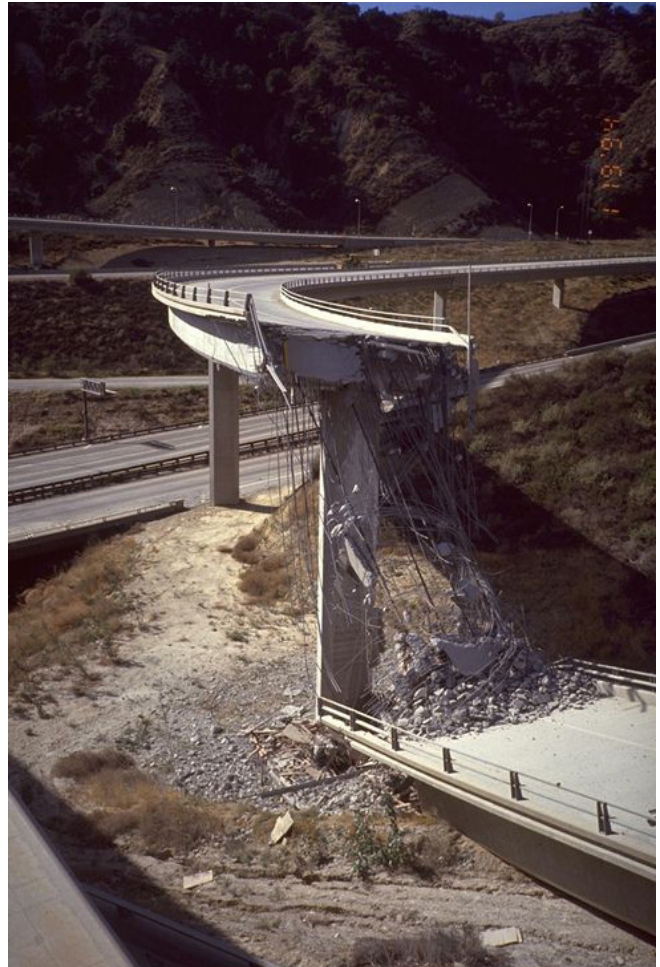
Figure 27. Following the 1994 M6.7 Northridge Earthquake in California, several freeway bridges such as this post-tensioned north to south connector ramp, completely collapsed. Heavily damaged and collapse of bridges that have not been seismically retrofitted may severely disrupt transportation and take years to demolish and rebuild. Photo: Guillermo Santana.
