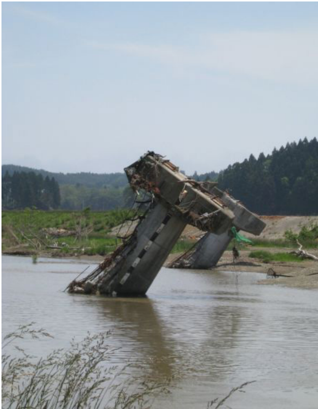
Figure 26. Tsunami waves following the 2011 Tohoku earthquake in Japan slammed into a pier supporting a rail bridge. The force of the tsunami waves washed away the bridge spans and heavily damaged the pier. Photo: Shideh Dashti.
