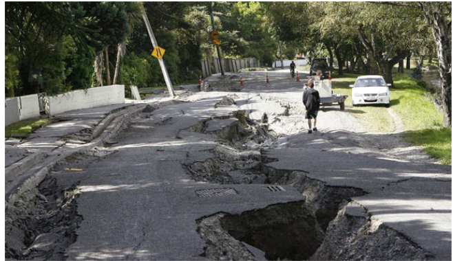
Figure 20. The 2011 M6.3 Christchurch, New Zealand earthquake caused high damage to roadways as a result of ground failure due to liquefaction. This type of damage may require the removal and replacement of existing pavement. Photo: David Hallett, HITRAC.
