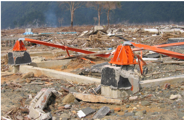
Figure 106. The 2004 Indian Ocean tsunami compounded communication infrastructure damage already caused by the earthquake, including completely knocking over cell towers. Widespread damage to communication systems can delay the response time of emergency services and leave survivors without crucial information. Source: USGS.
