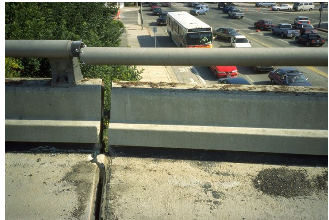
Figure 25. The 1994 M6.7 Northridge Earthquake caused low damage to a California highway bridge, shifting sections of the bridge and breaking a guard rail. Bridges with low damage should be operational and require only minor repair later. Photo: Mark Aschheim.
