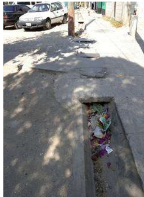
Figure 14. Trash accumulation in drainage ditches.
