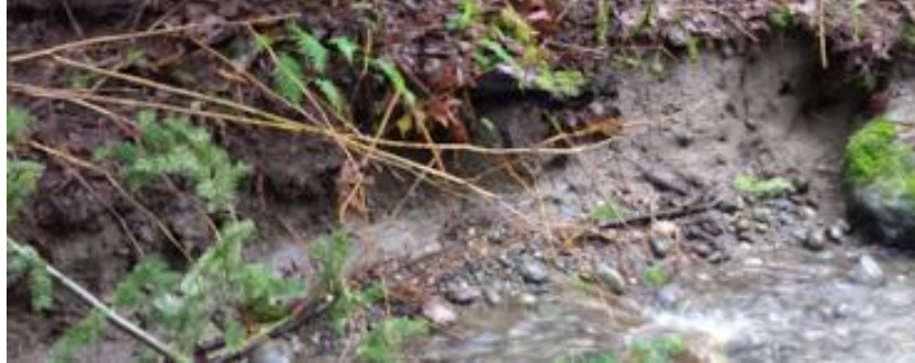
Figure 7. An undercut streambank to the left of the culvert inlet, where backwater pools during high flows, and erodes the streambank.
