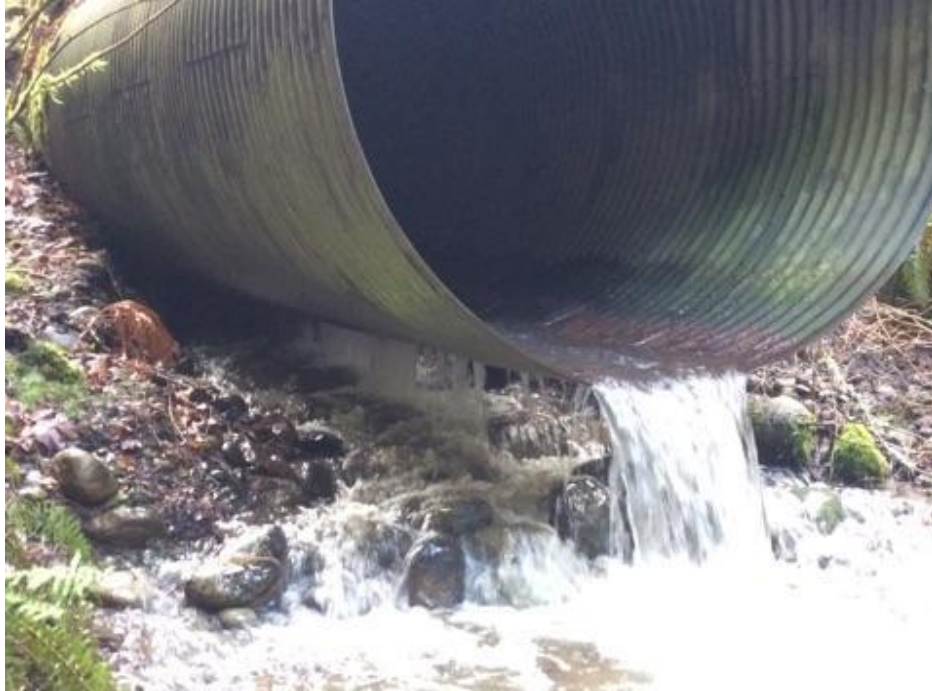
Figure 2. Water seeping from the rusting culvert bottom.
