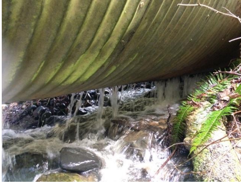
Figure 8. Water spilling out from the deteriorating culverts bottom, eroding the fill material below the pipe.
