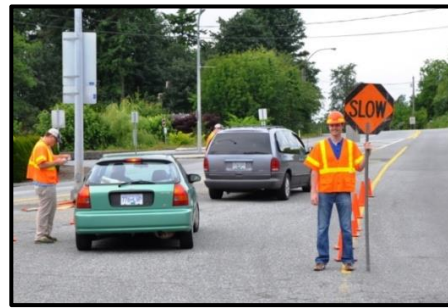
Surveyors conducting post-inspection surveys off of the main exit arterial NB at Lynden-Aldergrove.
