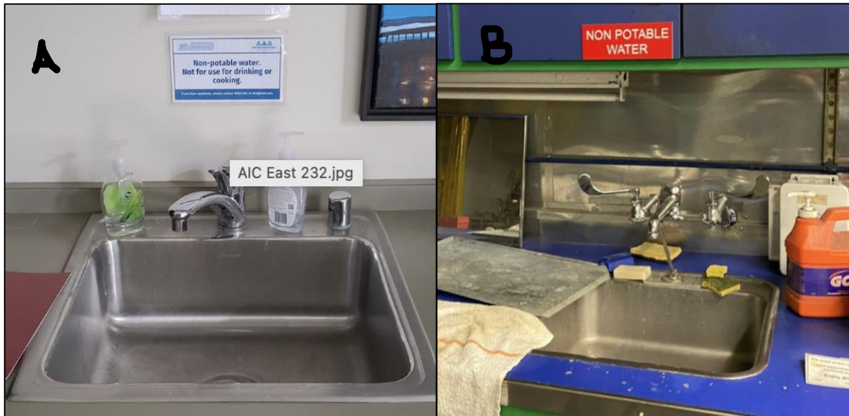
Figure 5. A. A sink in the Academic Instruction Center East, room 232, that has been temporarily signed as non-potable. B. A sink in the Physical Plant, room 212, that has been permanently signed as non-potable.
