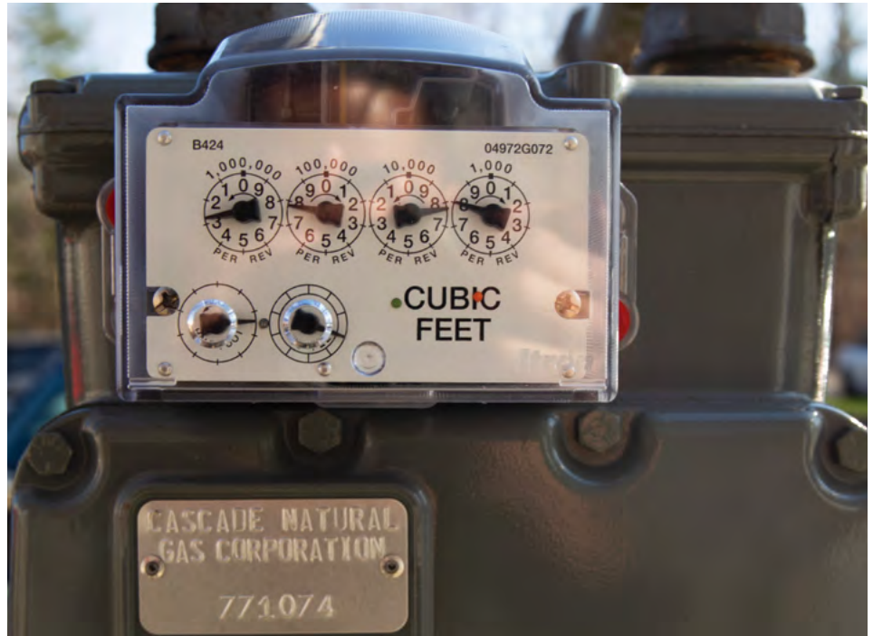
ABOVE: A natural gas meter at Barkley Village in Bellingham. If the task force’s proposals are implemented, this kind of energy infrastructure would no longer be used in Bellingham.
