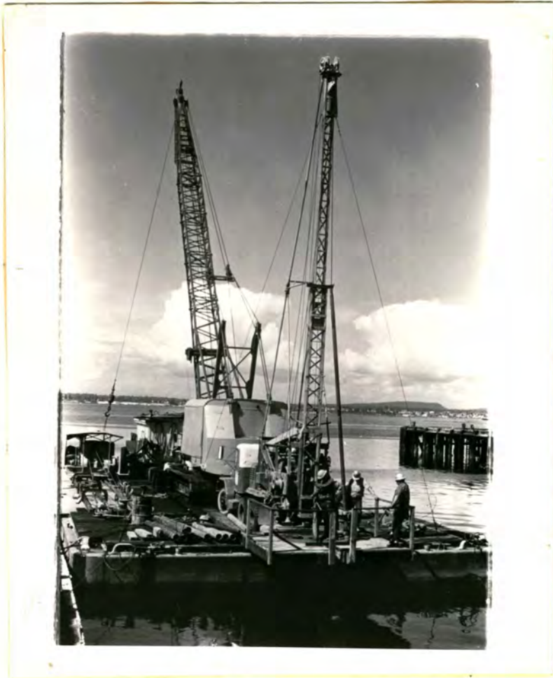
Fig.6 Drilling equipment rig mounted on Port of Bellingham barge for offshore drilling.
