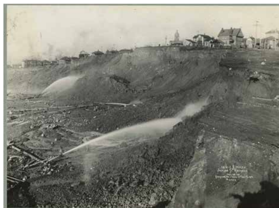
Figure 2. Regrading projects in Seattle sluiced over 200 thousand cubic meters of sediment into nearshore waterways. This photo shows hydraulic sluicing. Photo caption reads, “Lewis & Wiley, Inc; Jackson St. Regrade; Dec.28.08; Looking W. from 11th and King; #11752.” (Courtesy of City of Seattle Archives).
